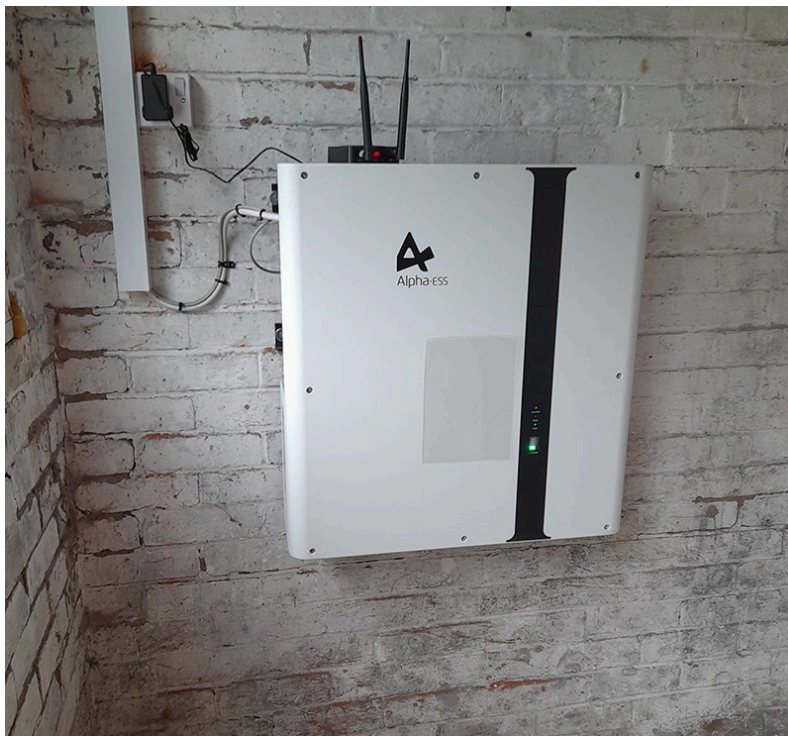
Figure 3.15 Installation of an Alpha ESS SMILE-B3 battery in an outhouse with a mobile router
